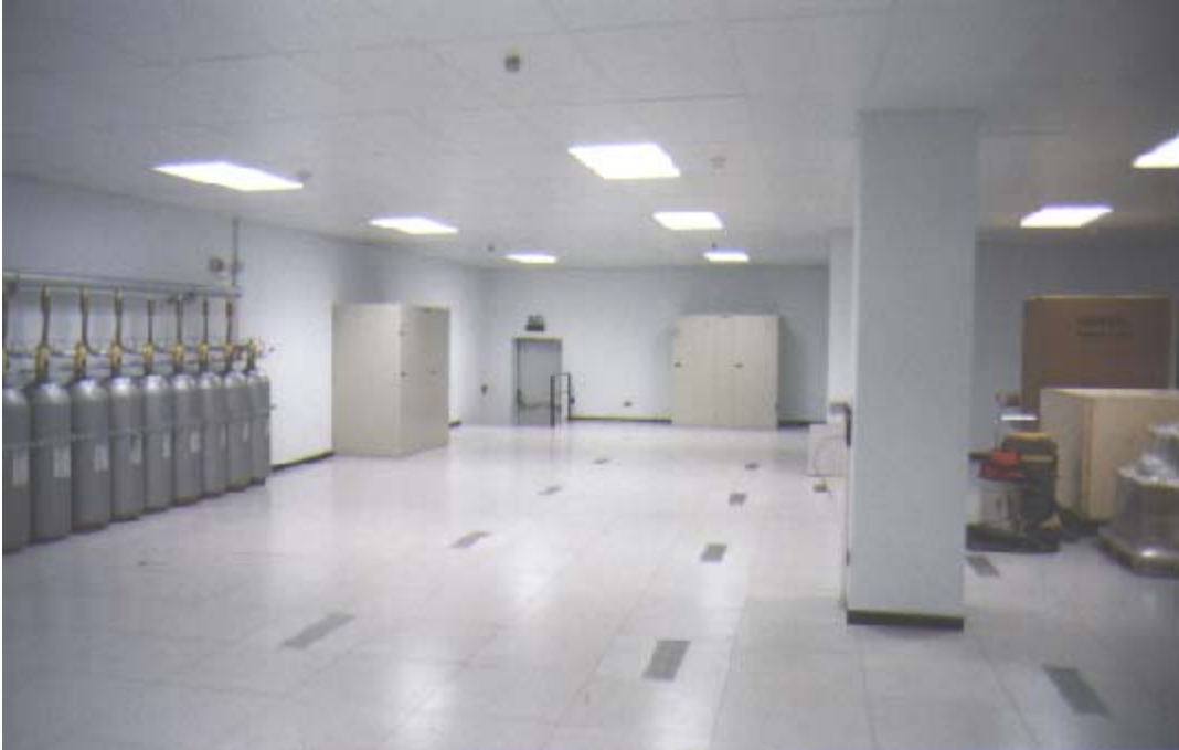
INTERIOR OF SWITCHROOM, AS OF DEC. 99
